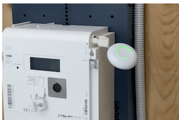
Figure 43 Example of additional P1 meter
